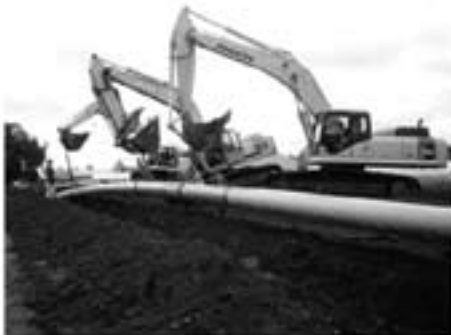
Natural Gas Mainline Aurora, OR
